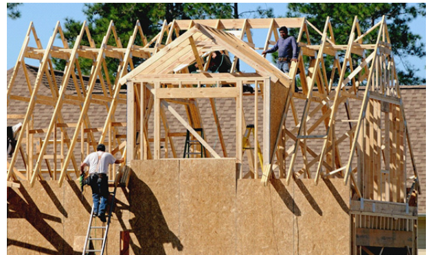
Construction crew works on a new home in Leland, N.C. Photo source: Associated Press
