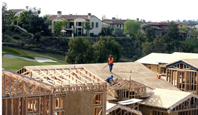
Workers install roofing material on a house under construction in Rancho Santa Fe, Cal.
